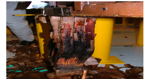
South Africa Transformer overheating 15 Transformers damaged
